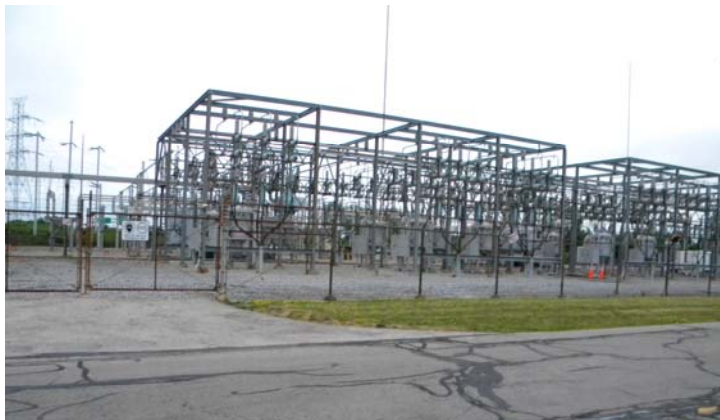
High voltage power substation at the University of Buffalo—where the abandoned bunnies liked to hide.
